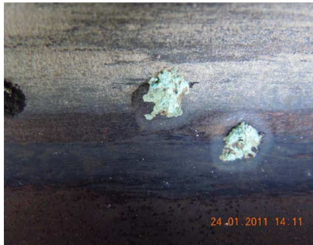
Figure 1: Typical Type 2 pitting corrosion product appearance on pipe experiencing hot water pitting corrosion. (Author’s collection)
