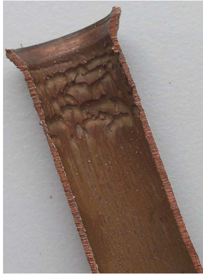
Figure 5: Deeply 'scalloped' pipe surface, typically near pipe joint. (Nicholas, courtesy of G. Moore, 2014)
