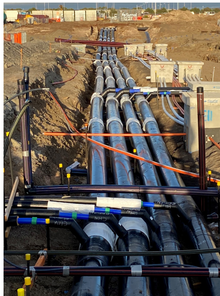
aquatherm blue pipe TI CHW and HHW systems installed in the trench
