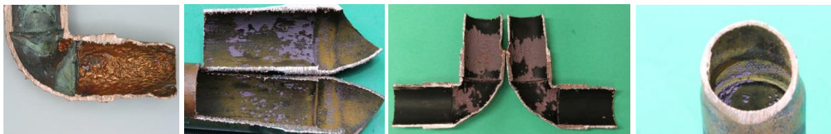
2) Erosion-corrosion in copper pipes
