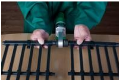
3) Push internal connection of the first grid into the (socket) heating tool and at the same time the external connection of the second grid onto the (spigot) heating tool.
