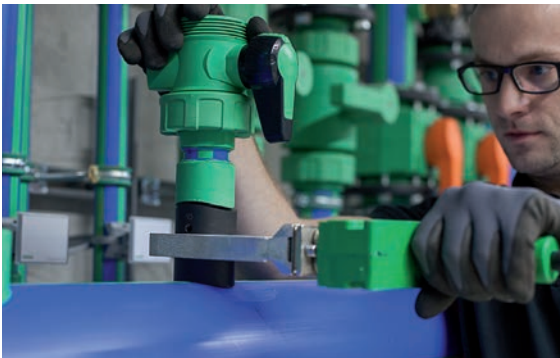
1. The aquatherm component unit is welded on the media pipe using special saddle welding tools.
