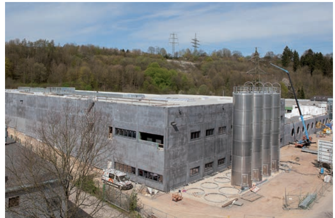
View from the administration building: Here, later on 12 silos will be placed for the supply with raw material
