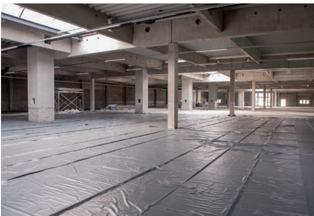
On the upper floor, the periphery for raw material supply is formed
