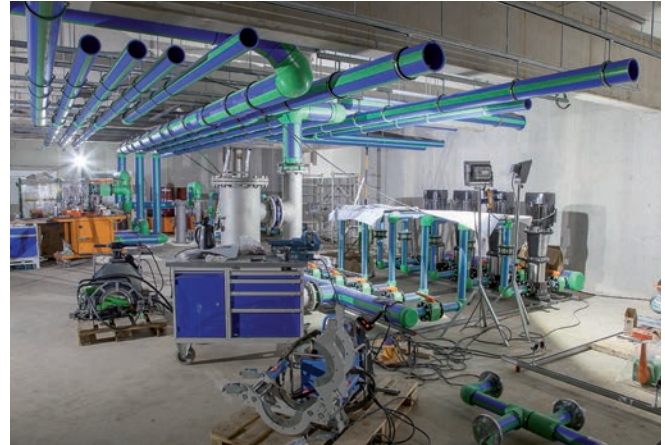
Cooling water treatment in the basement
